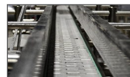
Conveyer Belt Monitoring
